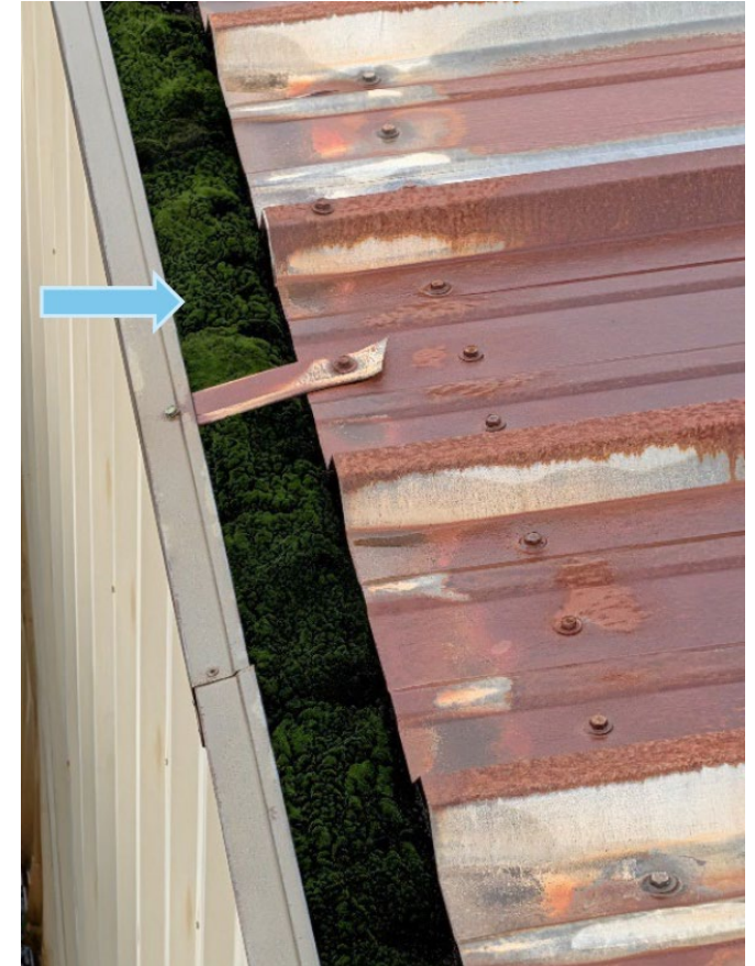
Clogged gutters and rusted panels
