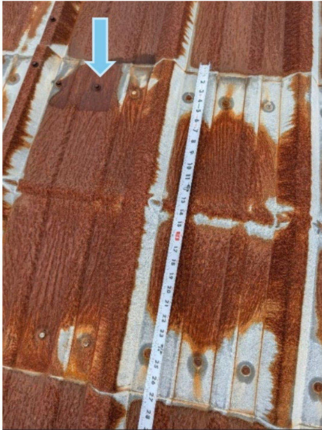
Rusted panels and corrosion around screw holes
