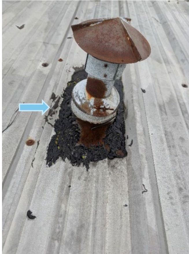
Deterioration and improper installation
