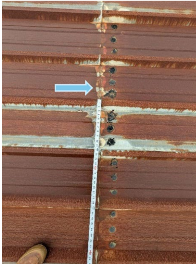
Signs of separation and deterioration
